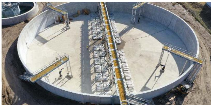
Circular Aeration Basin
