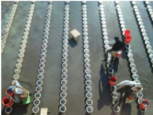
Membrane Diffuser Grid
